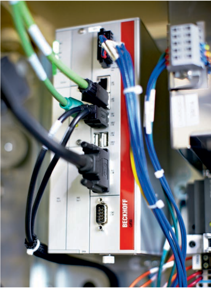
As a centralized multi-tasking controller, the C6930 Industrial PC drives the entire HyPET® HPP5 system, including PLC, motion control, measurement technology, communication to auxiliary devices, and all HMI functions.
